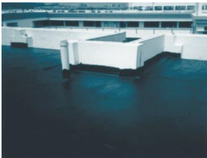
The old roofing system requires a waterproof layer on the main roof.
