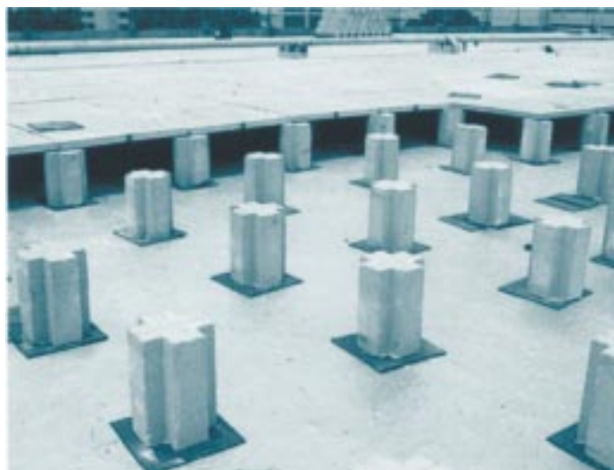
Stools are placed on the main roof to support the secondary roof.
